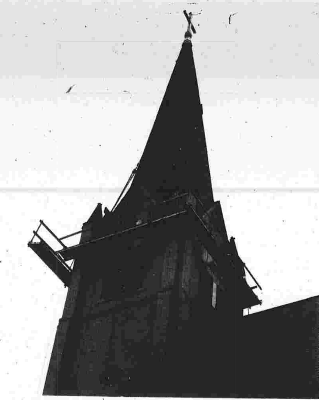
Workers at Emanuel Lutheran Church are repairing the steeple. It developed a few cracks and needs a bit of repointing (Herald photo by Pinto)
